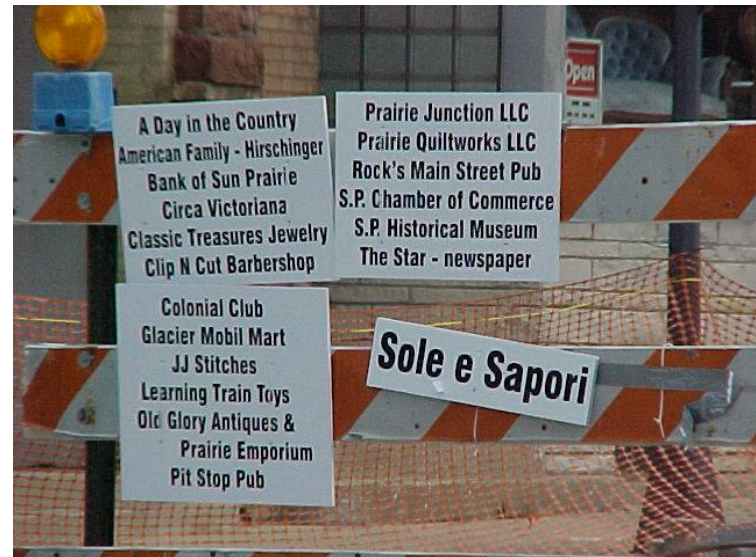
Bad example - individual names can't be read, lettering too small & cluttered, should not be on state barricade
